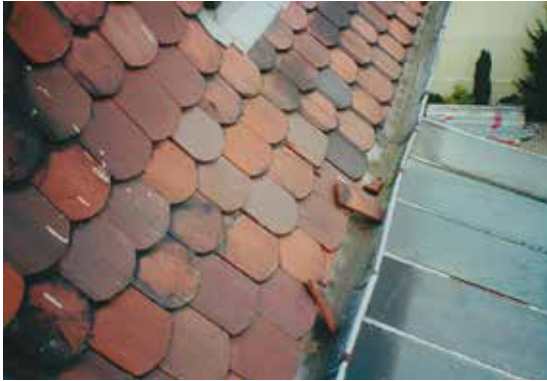
Lose Ziegel in Dachrinne
